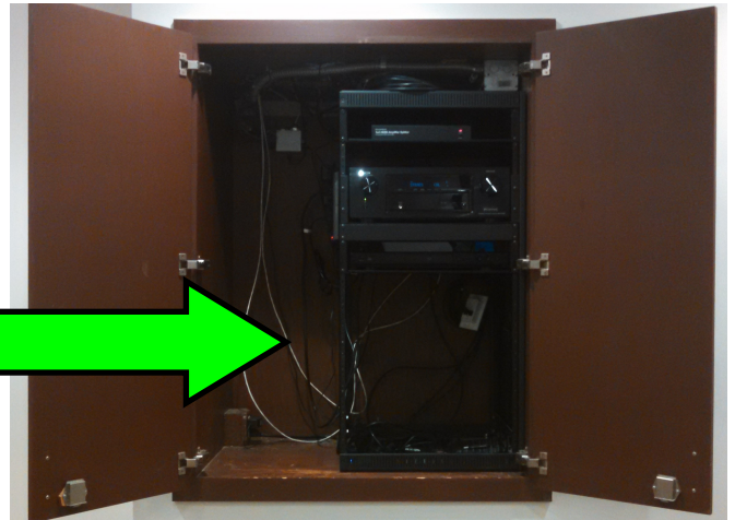
RACK IN G145 CABINET
